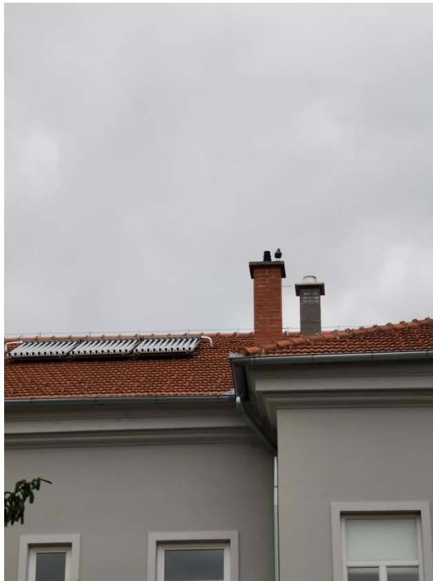
Figure 4.5 Solar collectors for domestic hot water heating on the administrative building
